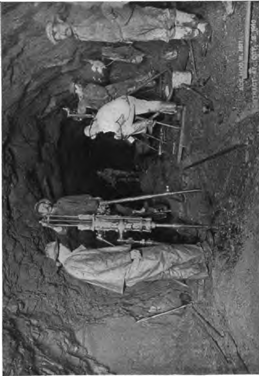
PLATE 119.—Contract 47. Tripod Drills on Bench which Usually Followed about 75 Feet Back of Face of Heading.
